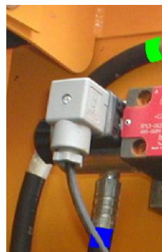
Wired DIN connector showing YELLOW/BLACK multicore cable from switch box in cab
